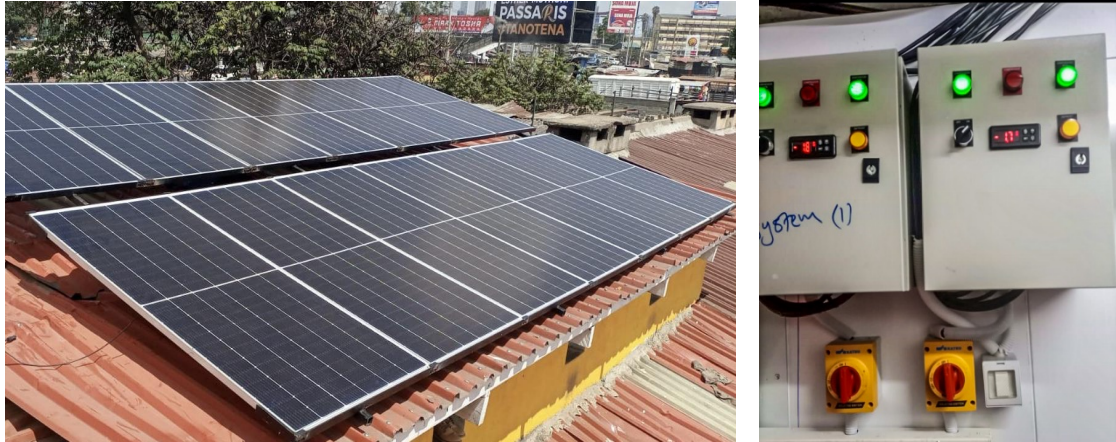
Figure 2: Unit 2 Solar-powered Freezer
